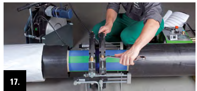
17. After the end of the cooling period the pressure is released at the hydraulic system. Then the mounting clamps are disconnected and the clamping device is removed.
