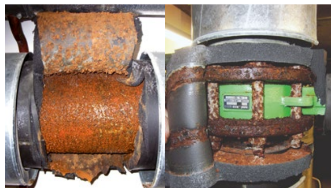
corroded steel pipes
